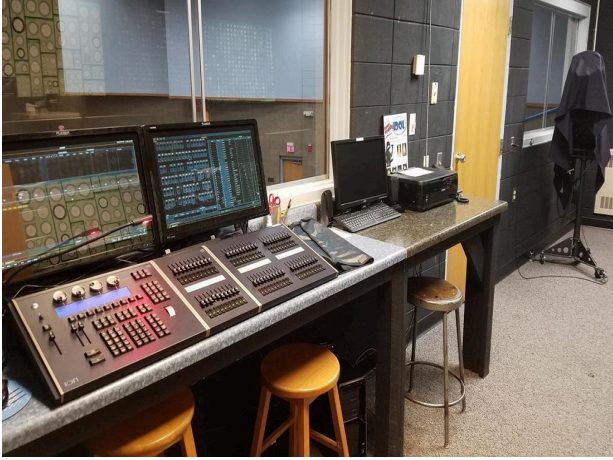
Lighting Control Booth
